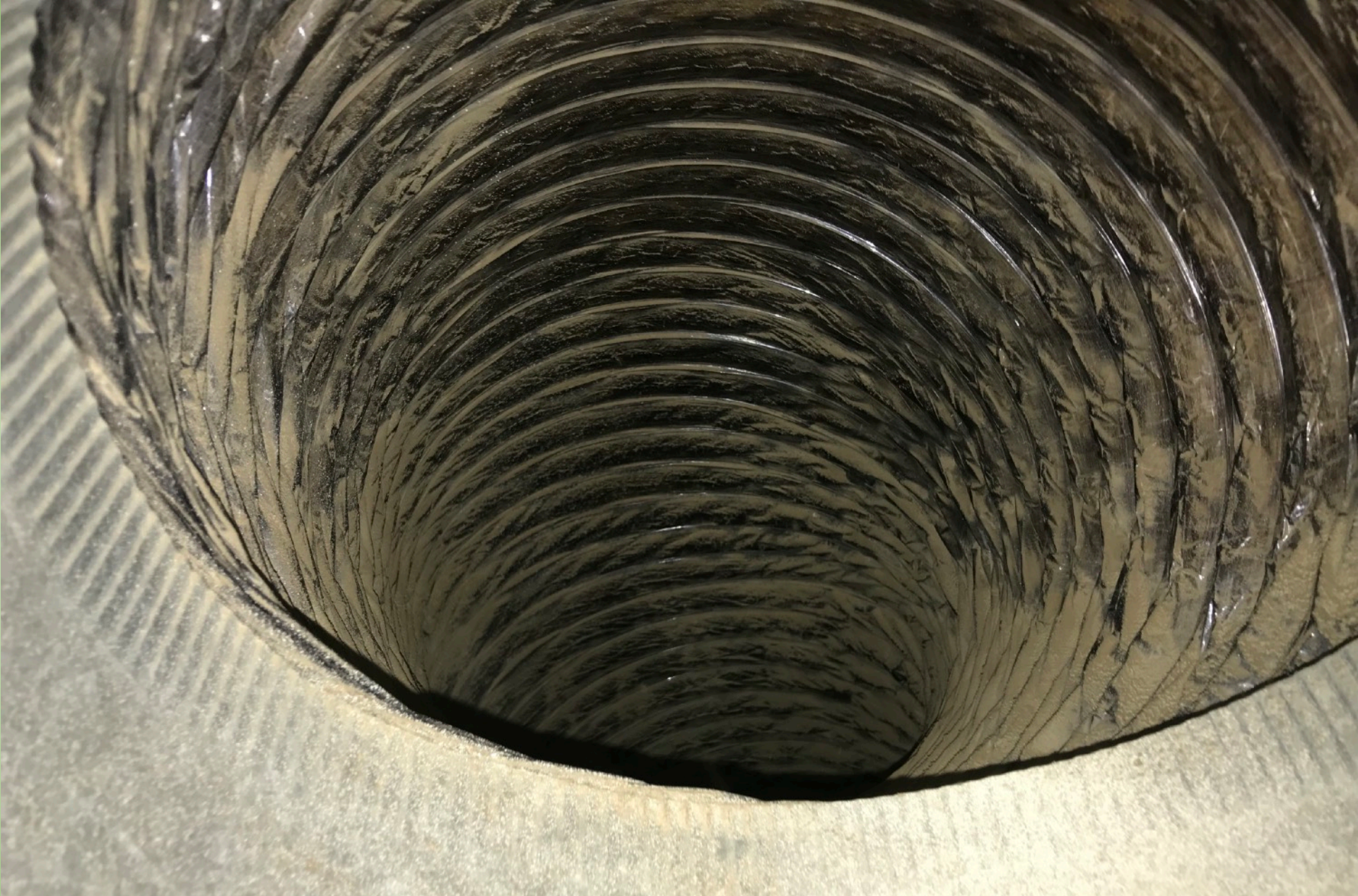
Cold-Air Return Dusty - Poor Filtration
