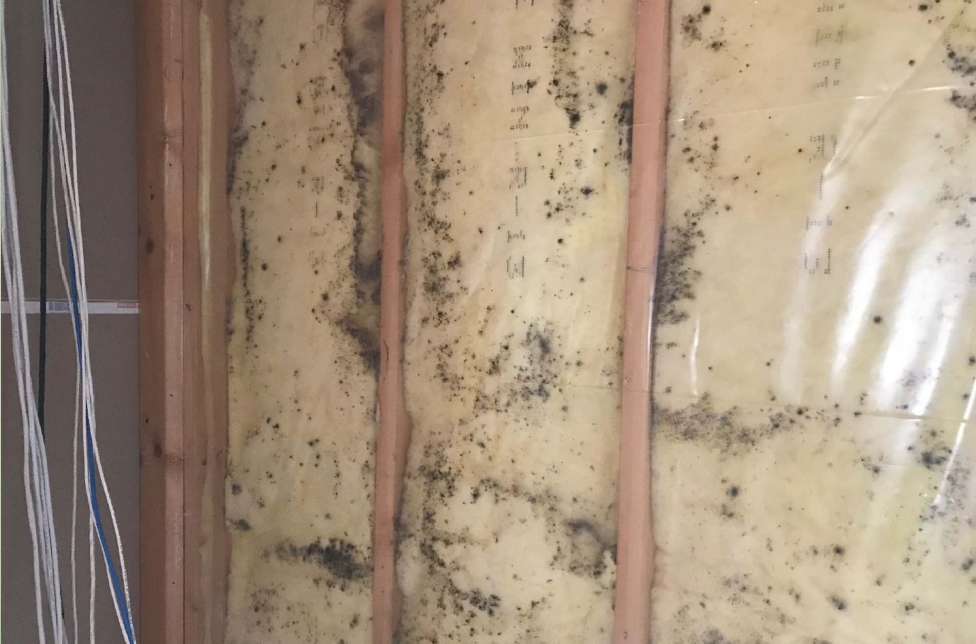
Mold on Insulation Under Wall from Poly-Barrier
