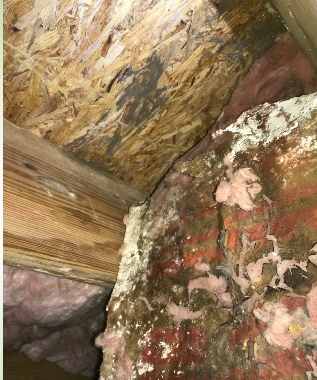
Mold in Crawlspace Under Insulation
